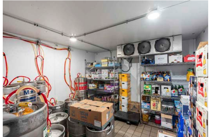
Upper Level - Walk-In Cooler
