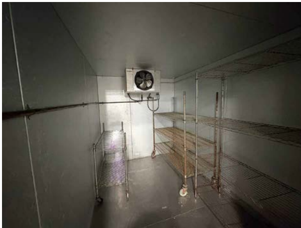
Main Level - Walk-In Cooler
