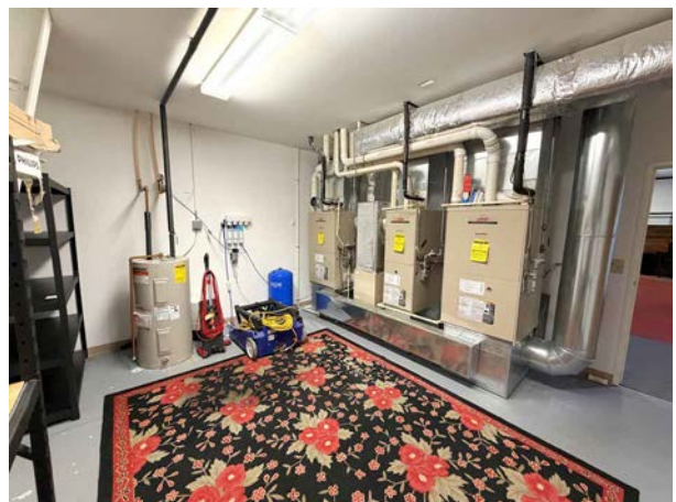
West Office - Mechanical
