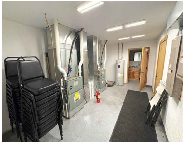
East Warehouse & Office - Mechanical
